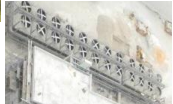
Air cooled condenser
