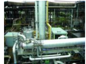
Steel Plant (Japan)
